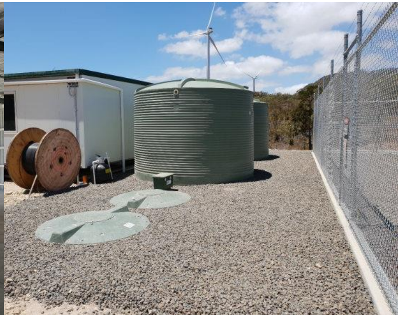
Site Control Building, water tanks and septic system installed
