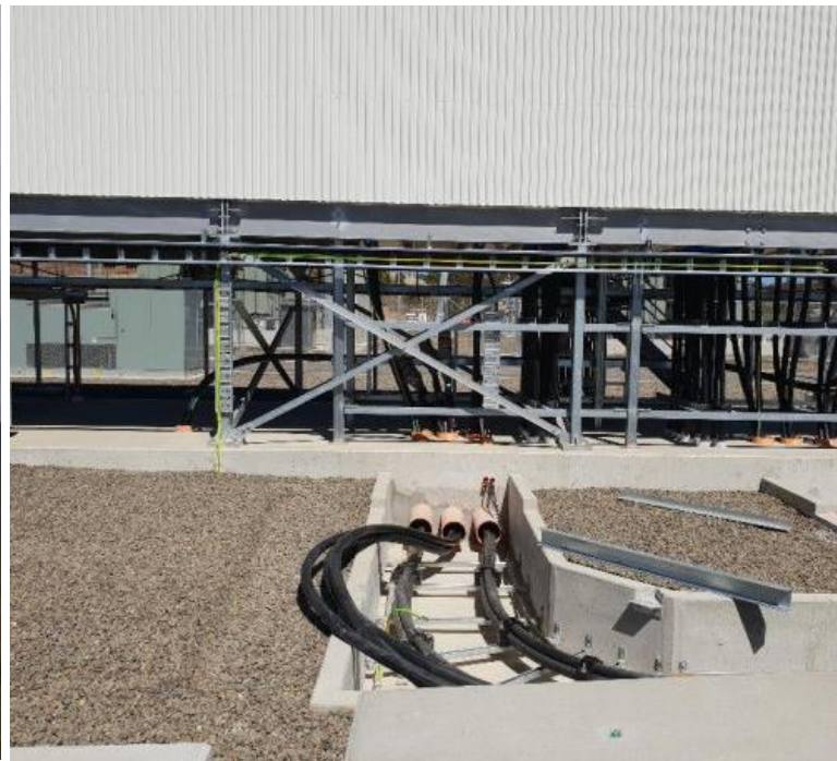
Cabling entry to control building
