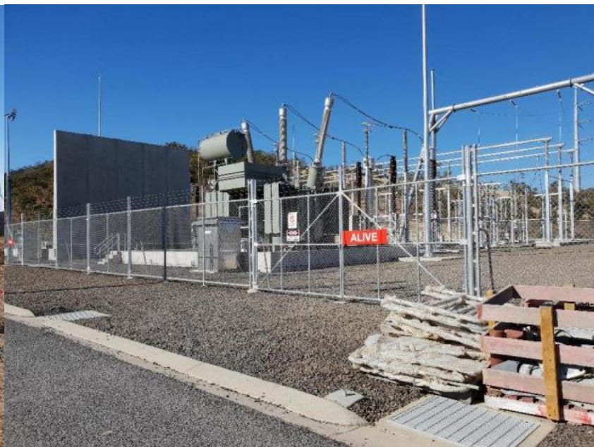
MEWF substation ALIVE
