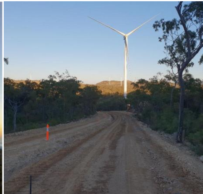
Cabling along roadway
