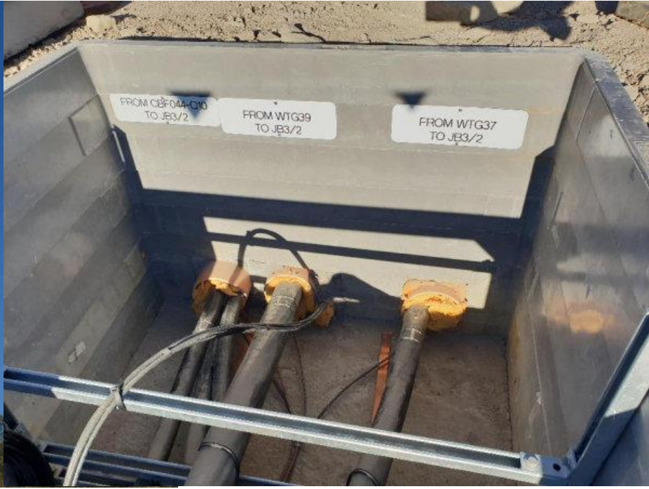
Cabling Junction Box
