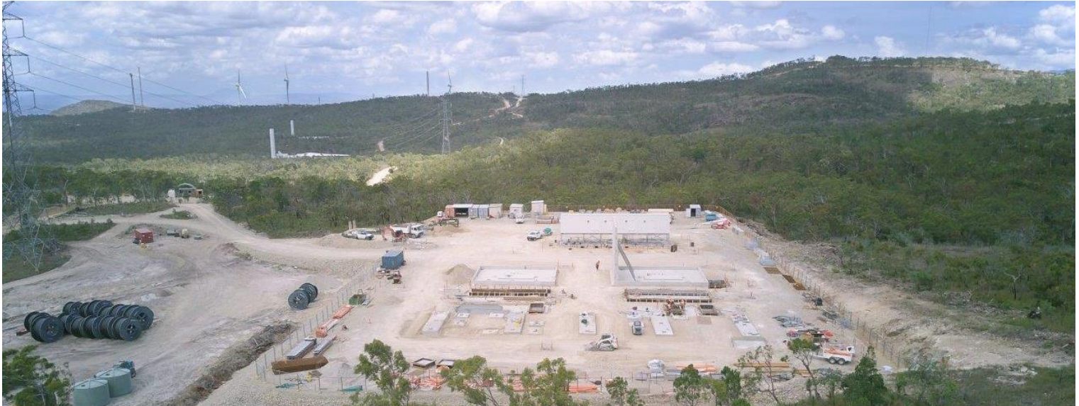
View of wind farm substation looking towards the east.
