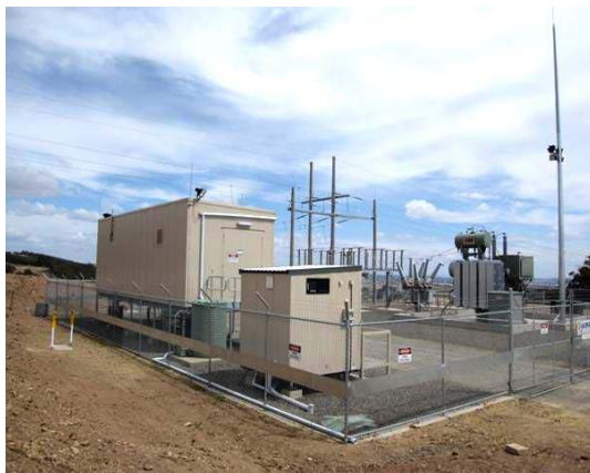
Plate 6 – Typical wind farm collector substation
