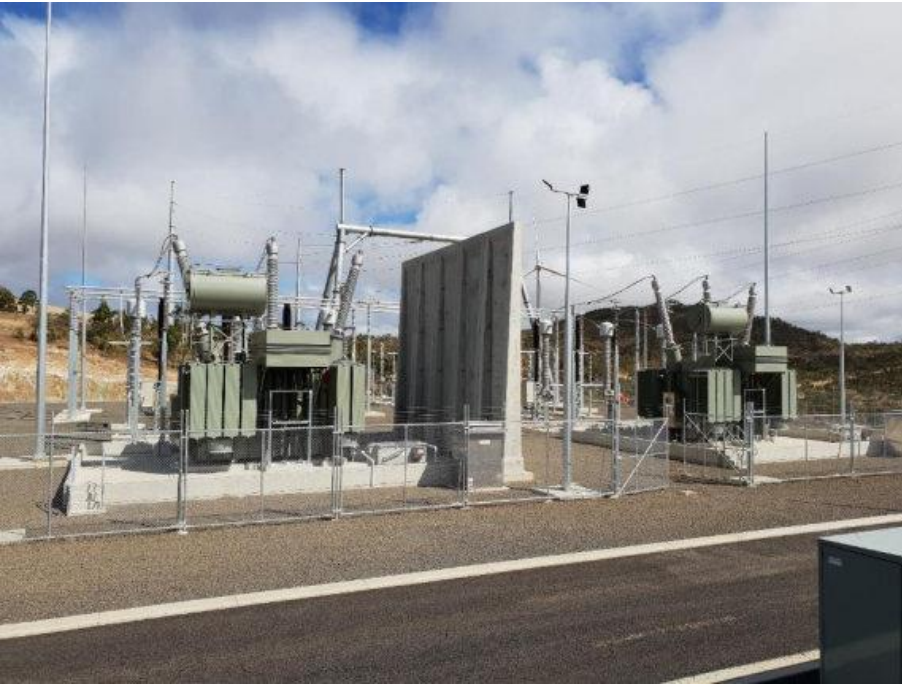
Wind farm substation
