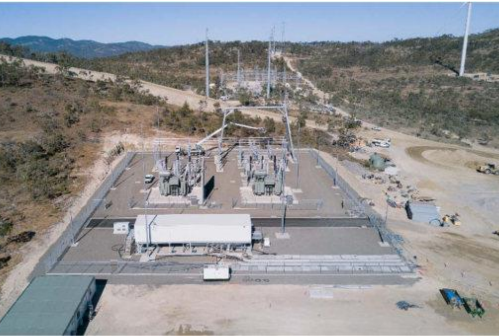
Aerial view of wind farm substation
