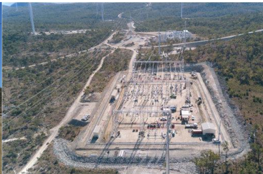
Aerial view of Powerlink Switchyard
