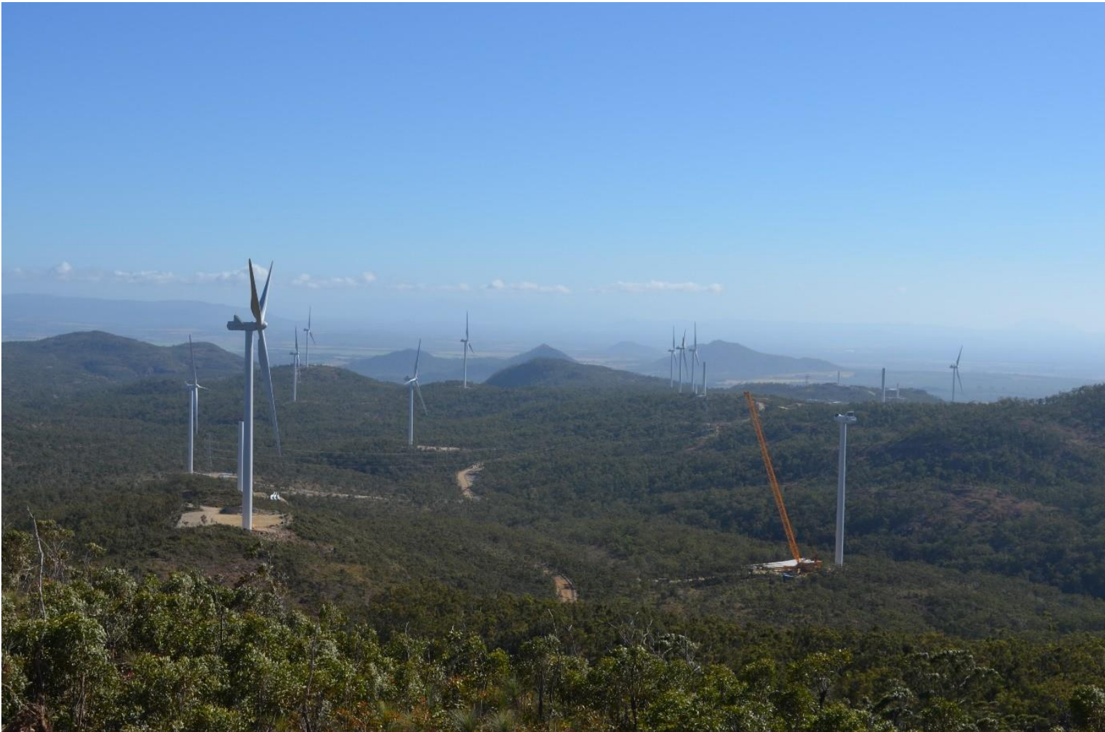
View from WTG32 looking north – complete WTG29 and installation of WTG26 in foreground
