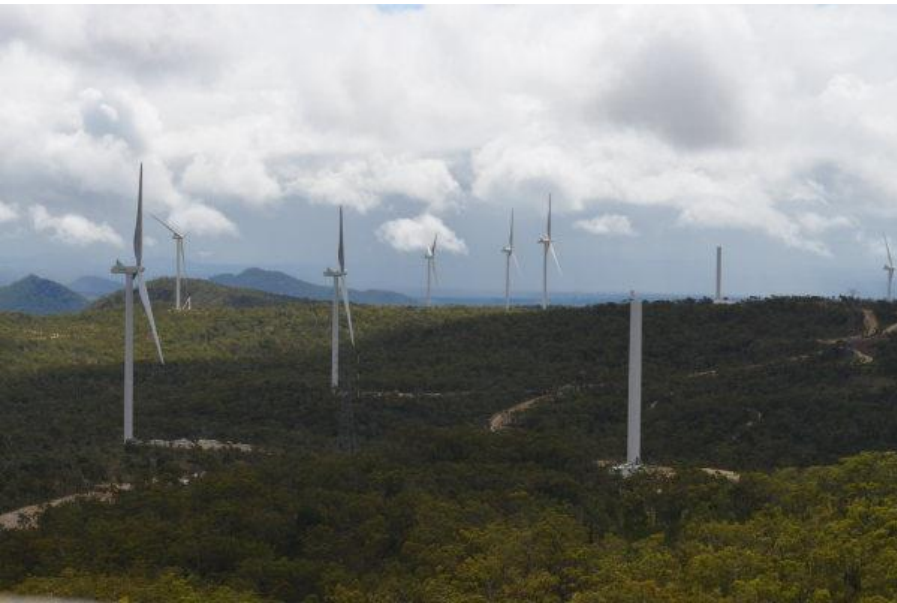
View NE from WTG24 (left front) and part complete WTG25 (right front)
