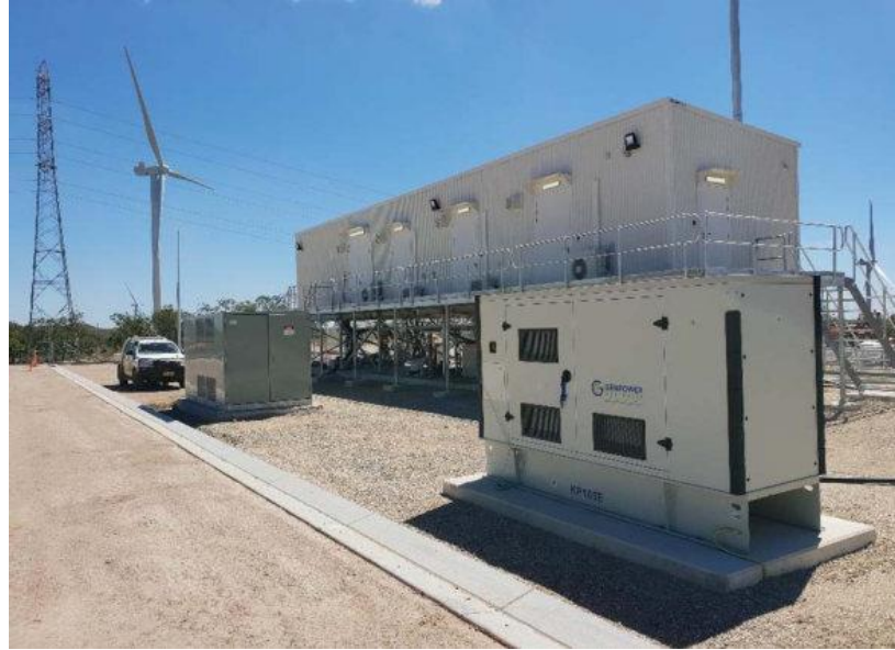
Wind farm substation building
