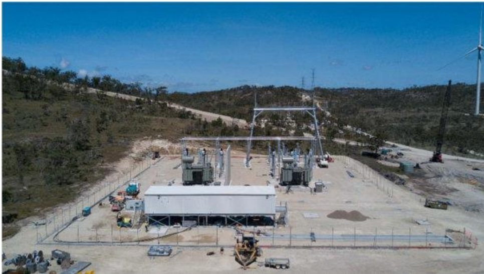
Wind Farm substation
