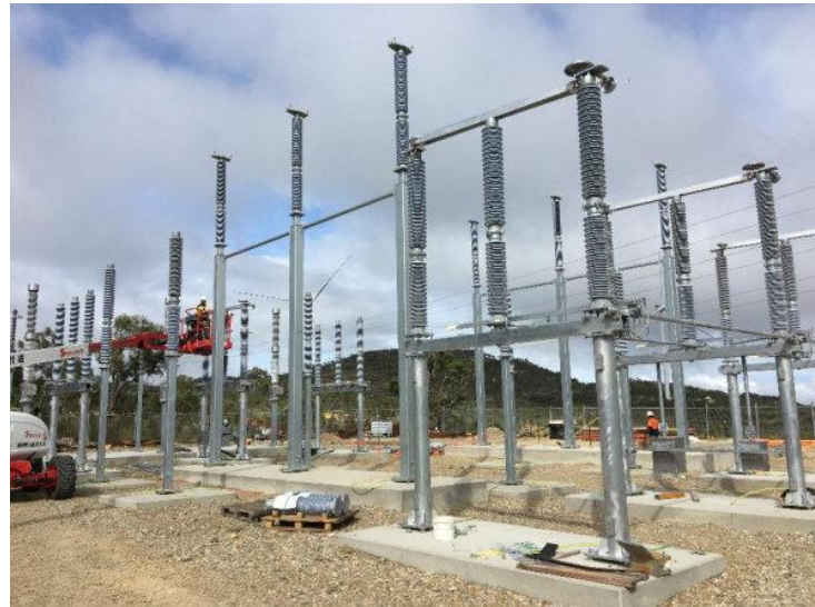
Overhead structures in Powerlink switchyard
